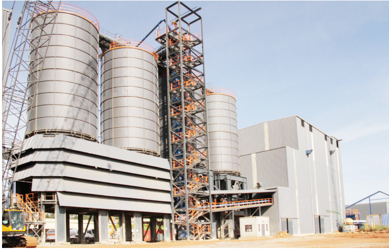
Latest state-of-the-art cement production factory at Namataba, 30km from Kampala
